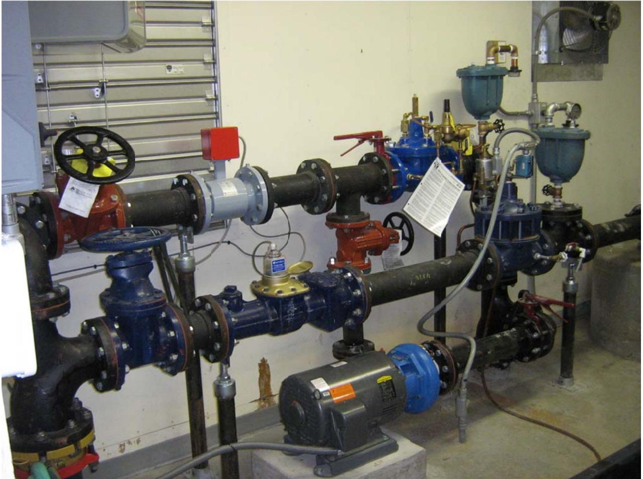
McKinney Water District Intertie
